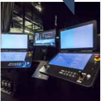
Sisteme de control
